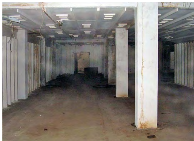
A recent internal view of the Llantarnam cold store showing the supporting pillars. Photo by 'MODman56'
